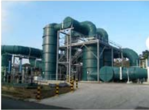
Odour Control Unit (East)
