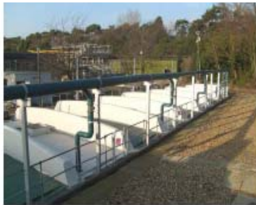
Storm Weir (East)
