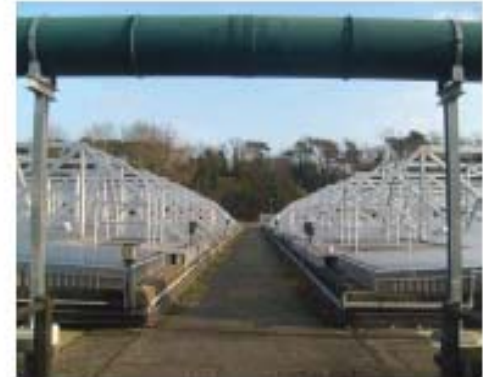
Storm Tanks 4 & 5 (East)
