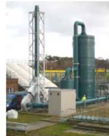
Odour Control Unit (West)
