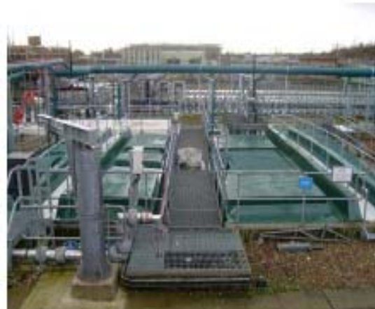
Cross Flow Grit Traps (West)
